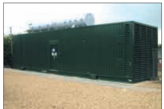
1825kVA set for Anglian Water – Turnkey design, supply, installation and commissioning by Yorpower
