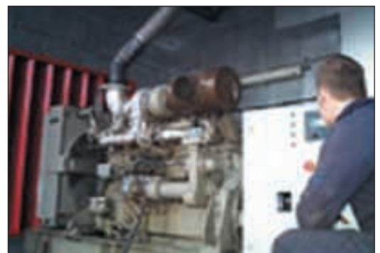
Generator on-test at our load bank facility
