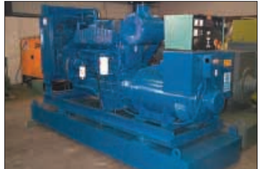
A completed 312kVA Cummins
